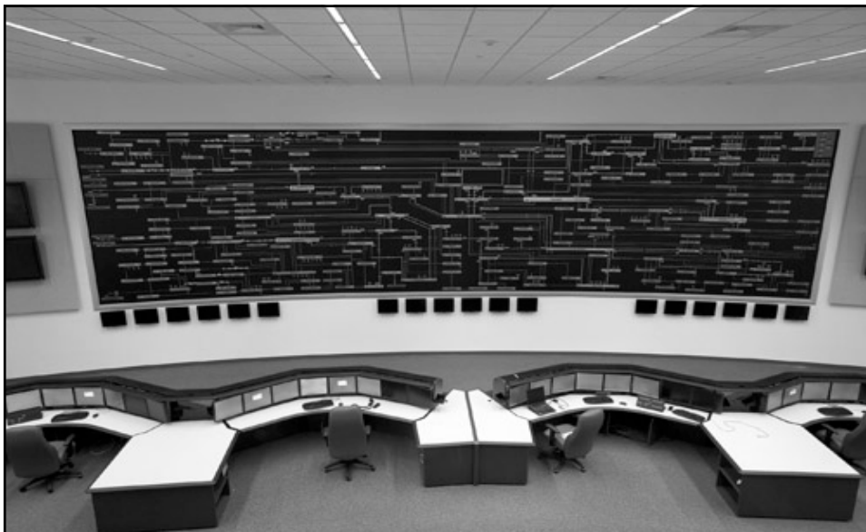
Wallboard: 9*3 array, 12 feet tall, 48 feet wide
